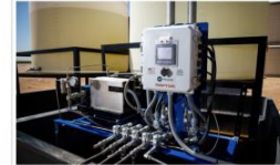
Chemical Injection multi-well control
